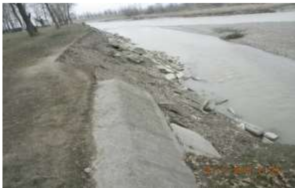
Figure 6 Upstream view of the study area on the Moldova River with erosion zones in the riverbed and bank (photo: Luca M., year 2014).
