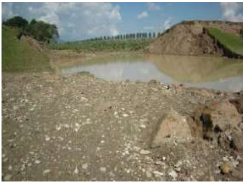
Figure 10 Horodnic Dam 1, Suceava County, 2008 - dam body degradation (CTM, 2010)
