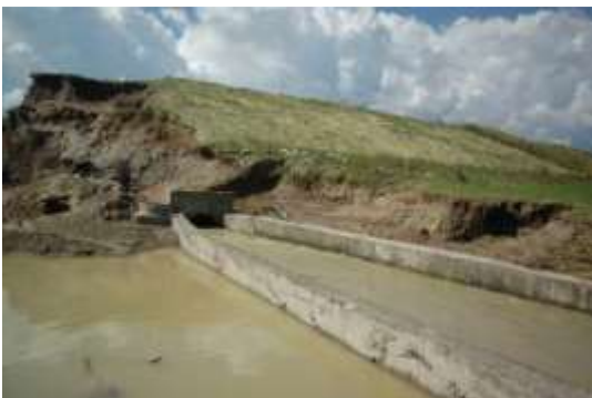
Figure 12 Horodnic Dam 2, Suceava County, 2008 - bottom emptying degradation (CTM, 2010)
