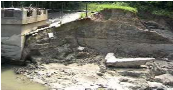
Figure 3 Crujana Dam, Suceava County, 2010 - breach through the dam, (ABA Siret, 2010)
