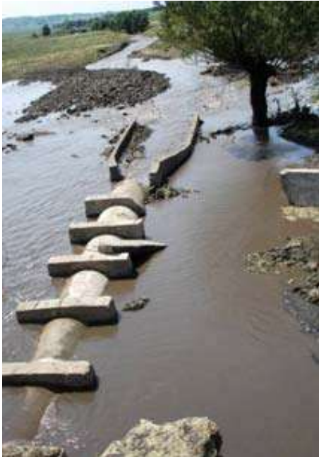
Figure 8 Grănicești Dam, Suceava County, 2010 - bottom emptying degradation (CTM, 2010)
