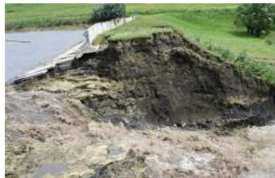
Figure 7 Grănicești Dam, Suceava County, Year 2010 - breach in the body of the dam (CTM, 2010)
