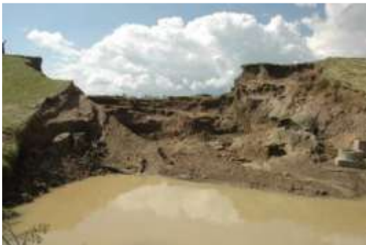
Figure 11 Horodnic Dam 2, Suceava County, 2008 - dam body degradation (CTM, 2010)
