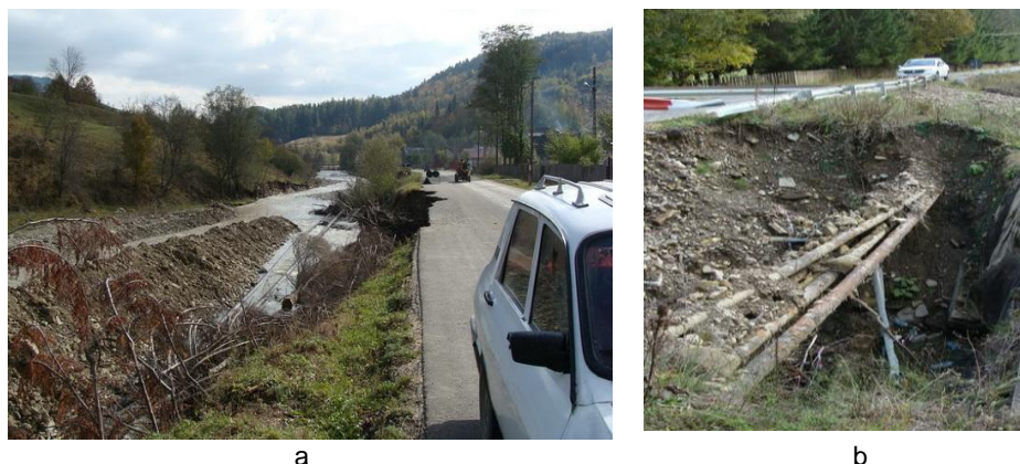
Fig. 2 Tazlăul Sărat river pollution risk zones: a - oil pipelines exposed by floods in June 2016; b - oil pipelines uncovered by the river infiltration stream (Avram, 2016).
